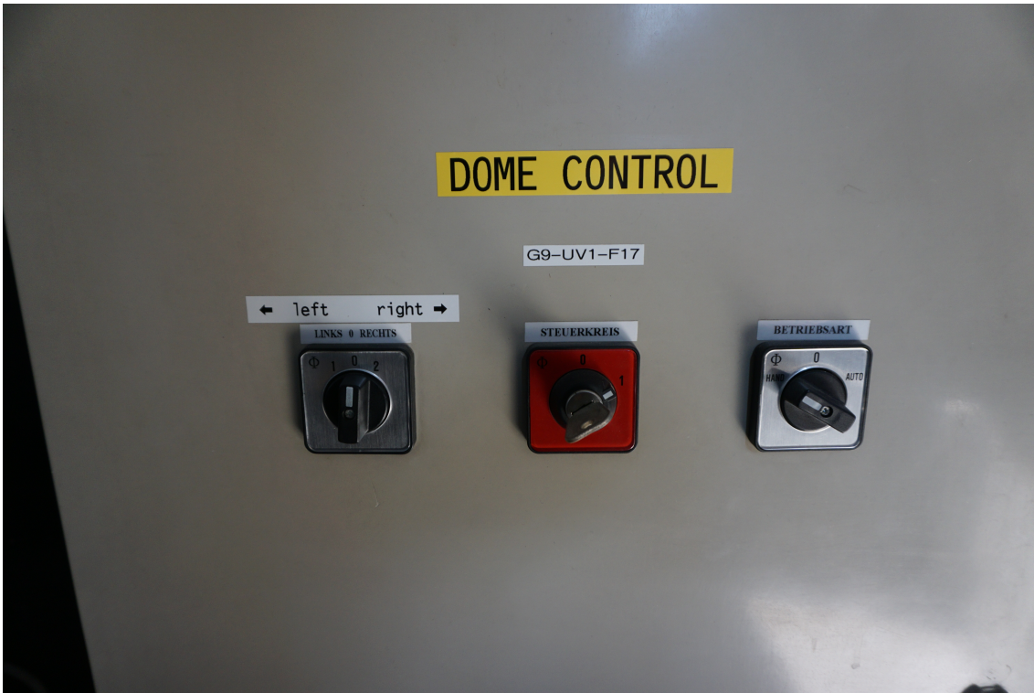
Figure 1: Switches for the rotation of the dome.
