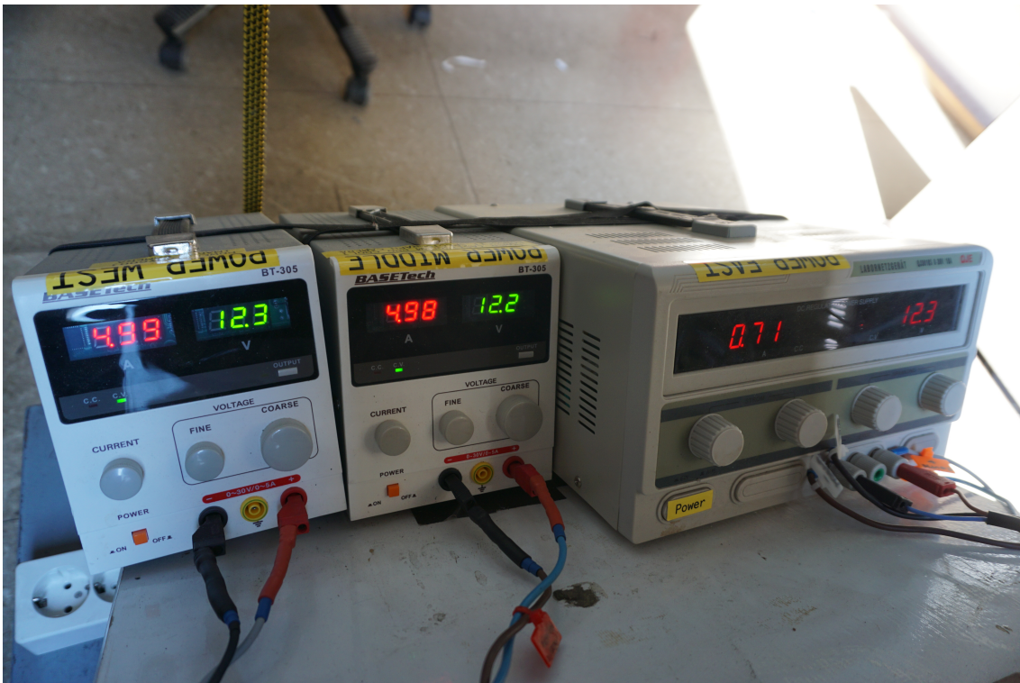
Figure 9: Power supplies of the mount, focuser and instruments within the dome.
